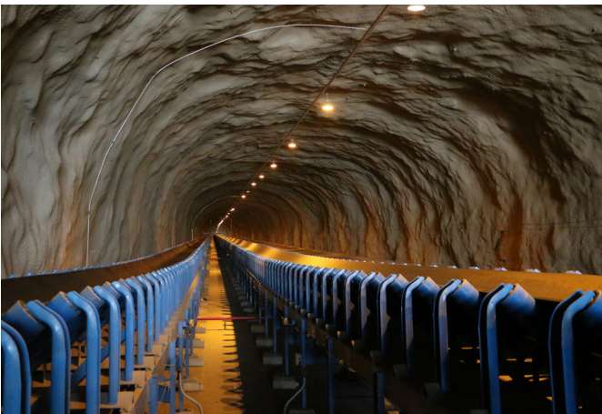
Sophisticated subterranean conveyor belt running 1.8 kilometres.
